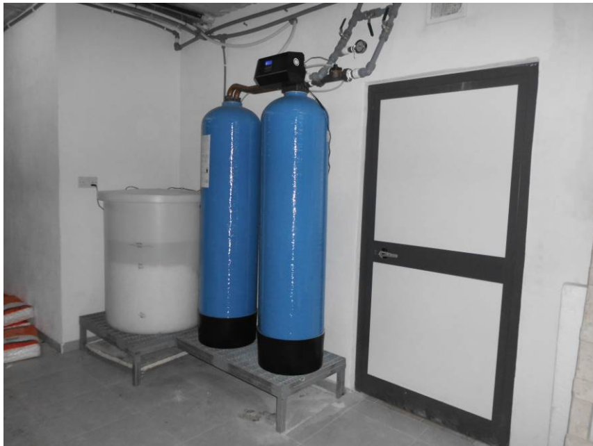
Photo 26: Water purifiers for kitchen use.
