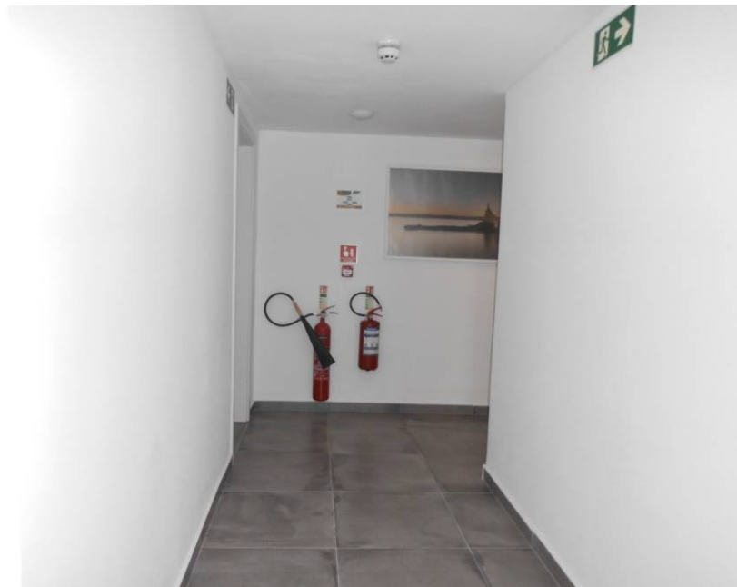
Photo 30: Firefighting facilities via dry risers.
