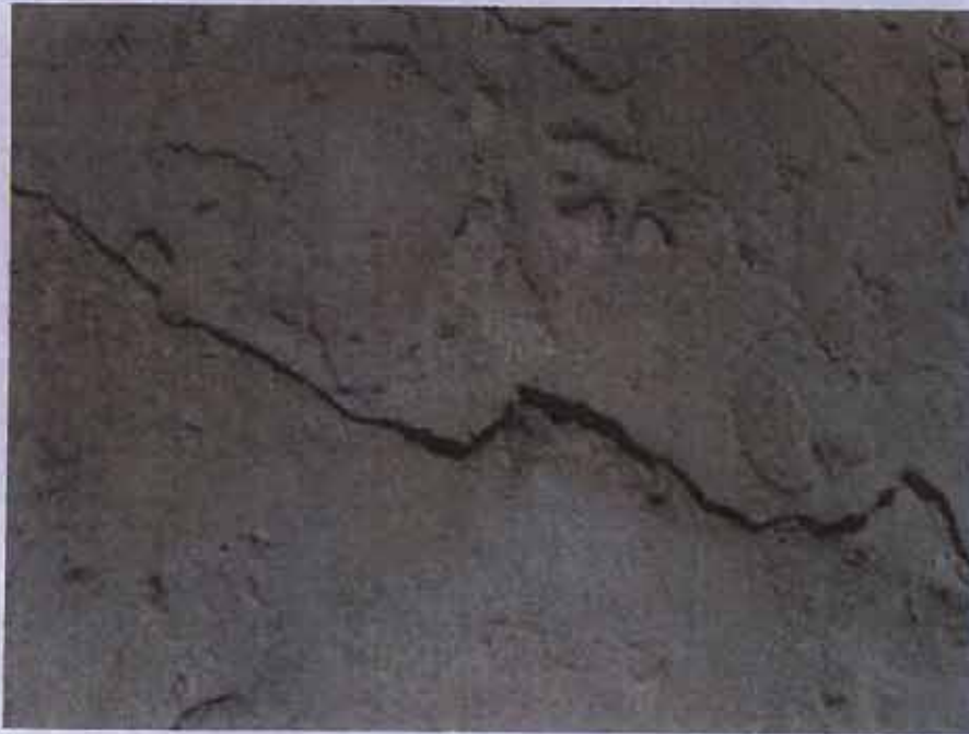
The south-east (front) façade – exfoliation.
