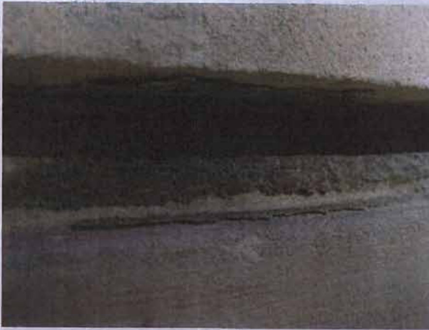
The south-east (front) façade at the porte-cochere – black crust.
