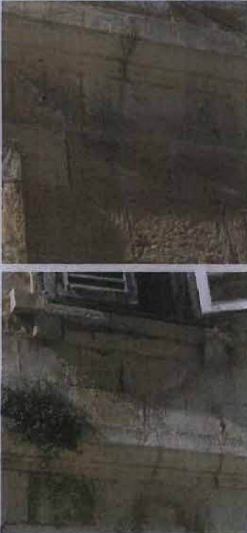
The historic stables – efflorescence and differential erosion.
