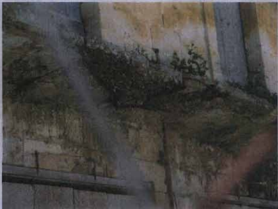
Historic stables – biological growth and the bad existing condition of the balcony.
