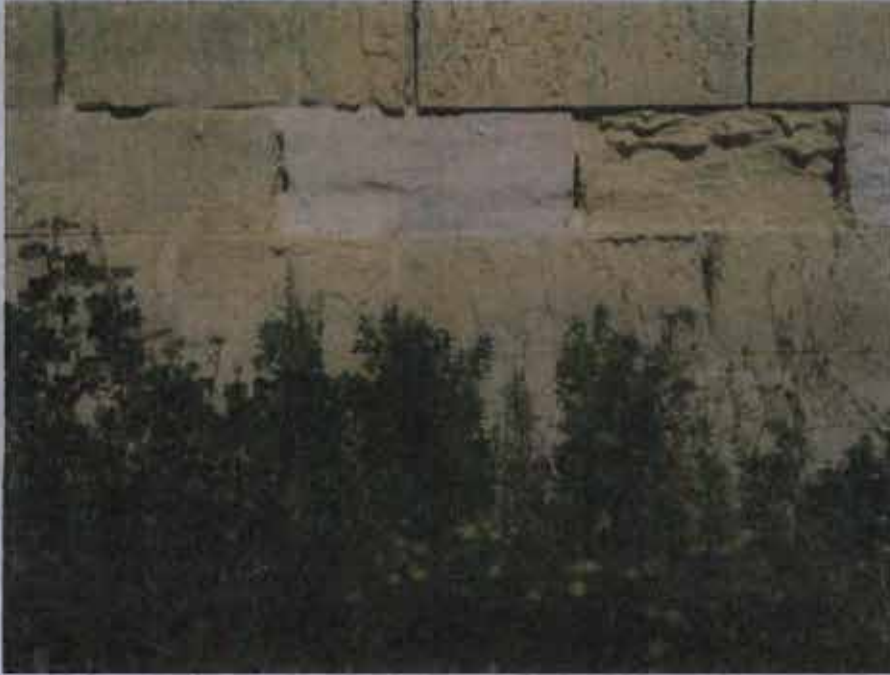
The historic stables – vegetation and surface erosion.
