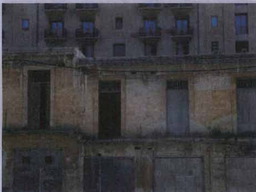
Historic stables – discoloration.
