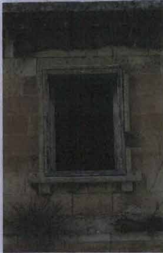
Figure 10: Photo showing bad detailing of timber frame
